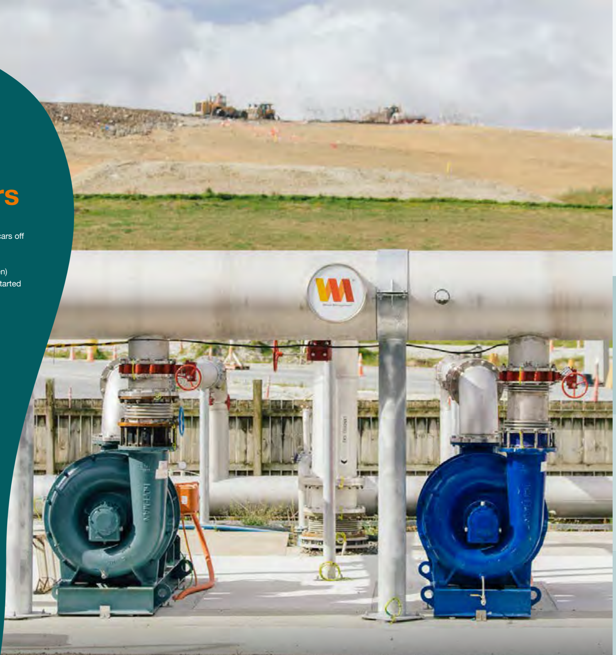
Gas capture at Redvale Landfill & Energy Park to supply to the generators, evaporators and neighbouring greenhouses.
