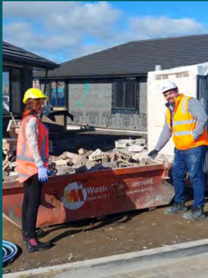
Site Manager Terence Beach and Stephanie inspect uncontaminated cleanfill bins at a Summerset Pohutakawa Place construction site.
